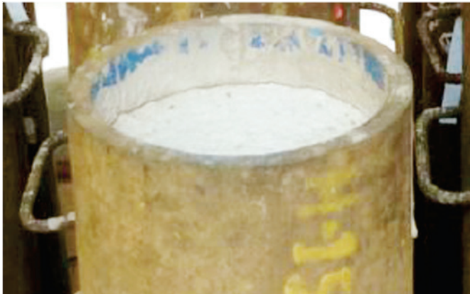
Figure 4 Detail of 50 mm void left during concreting
